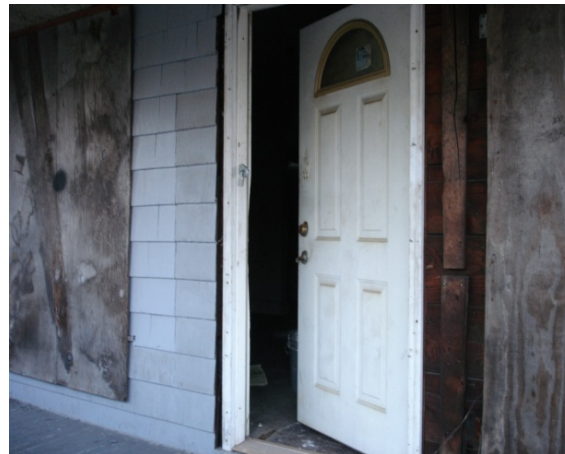
Padlock on front door broken – open to casual entry
